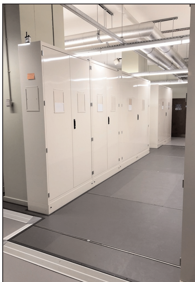
Figure 5: Compactor cabinets on the raised floor in the new store.
